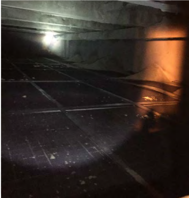
Wygen 3 U5 Top Layer with IGS Secondary LPA Screens
